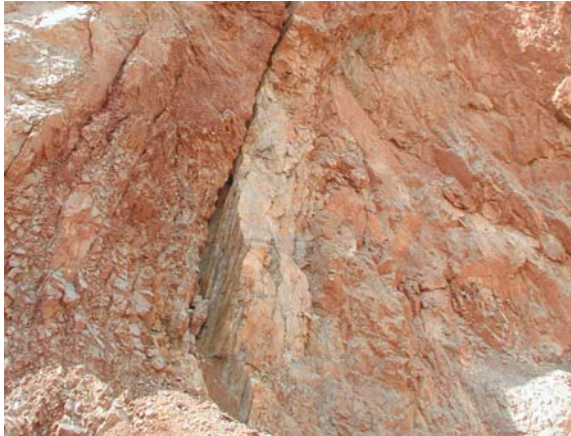
Fig. 26. Fault plane 209/73° with mullions at the documentary point 7-3 on the 7th storey.
