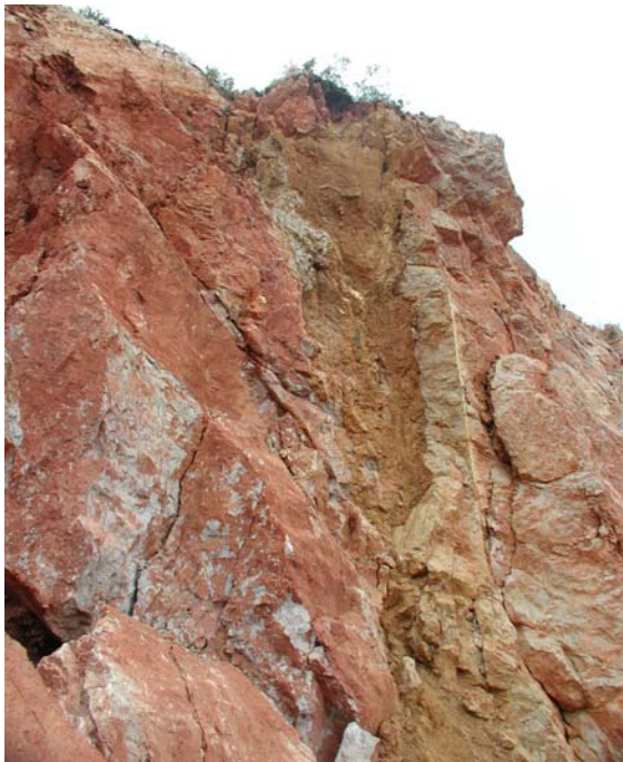
Fig. 49. 15 m deep sink filled by limestone blocks with clayey matrix on the 9C storey.
