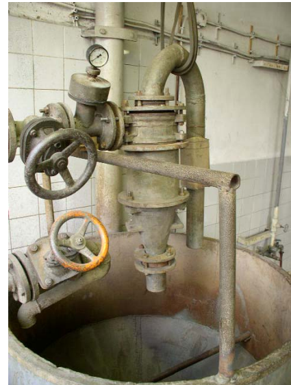
Fig. 2. Hydrocyclone station – real view.
