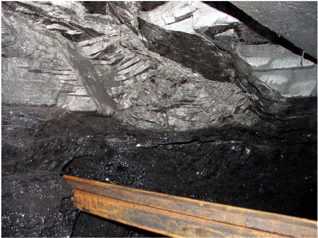
Fig. 9. Tectonic ramps and slicken-sides (mirrors) corresponds to thrust zone in the roof of Seam No. 30 (634) – Lower Suchá Member, ČSM Mine. Photo R. Grygar.
