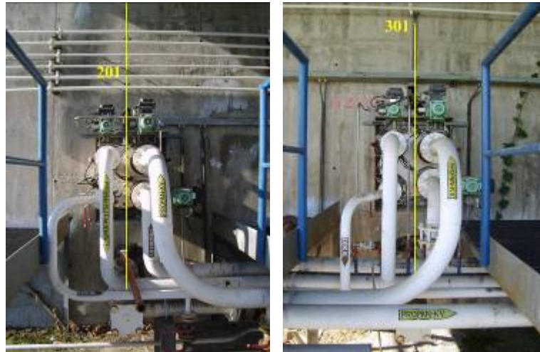
Fig. 4. Detail of the technological sector of the both of reservoirs PZ1 a PZ2.
