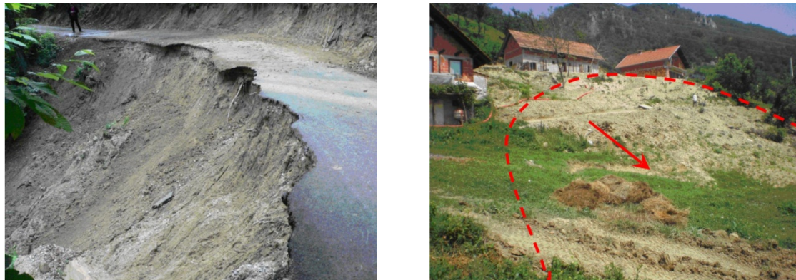
Fig. 2. Typical landslides in the Bednja area: 2A) Most frequent appearances at road bends; 2B) Often landslides will happen beneath houses.
