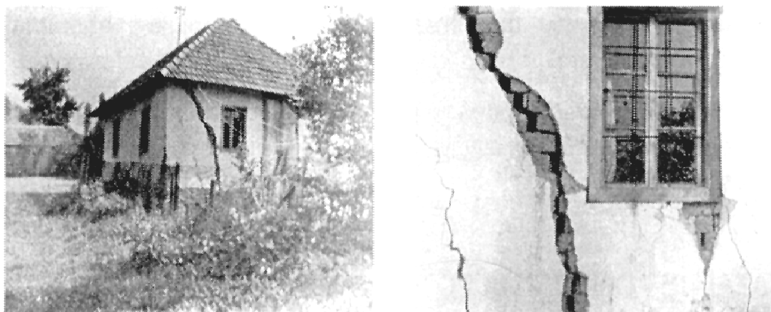
Fig. 6. Examples of damages to a private building caused by a terrain deformation.
