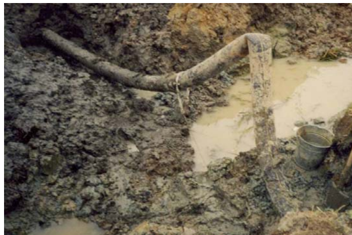
Fig. 6. Deformation of medium pressure gas supply pipeline PE Ø160 [3,15]
