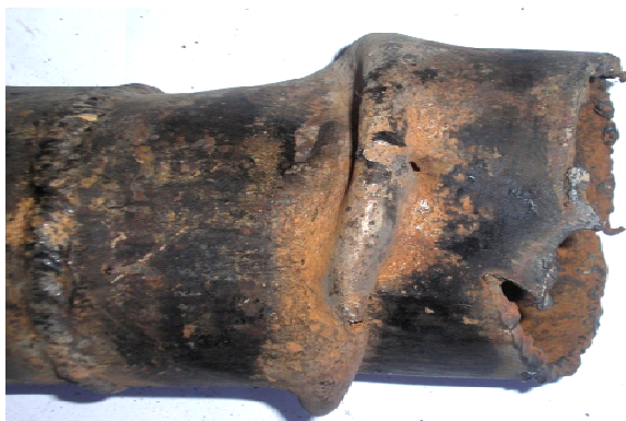
Fig. 3. Damaged section of steel pipeline \text{Ø}100 - folding of wall, damaged insulation, corrosion pits and holes [15].
