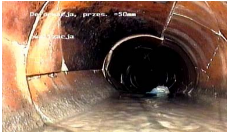
Fig. 5. Damage of stoneware sewer [12].
