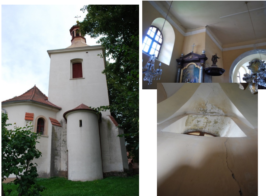
Fig. 1. Church at Světí near Hradec Králové, on the right: examples of failures in the church (photo: Kaláb).
