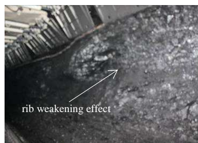
Fig. 12. Status of the wall after a reduction in the setting load.
