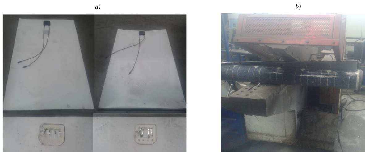
Fig. 10. a) Removed aluminium frames and junction boxes, b) PV modules cutting into two halves.
