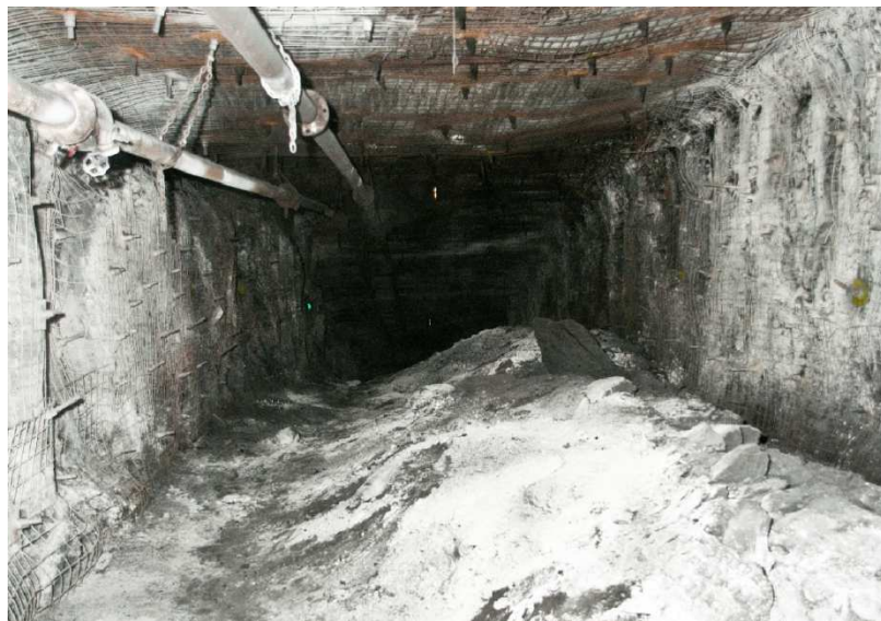
Fig. 5. Photo-documentation on floor swelling in the working
