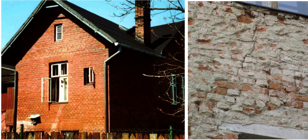
Fig. 11. Two examples of cracks in buildings damaged by vibrations in the surrounding of open pit Nástup Tušimice Mines. (Photo: Kaláb).
