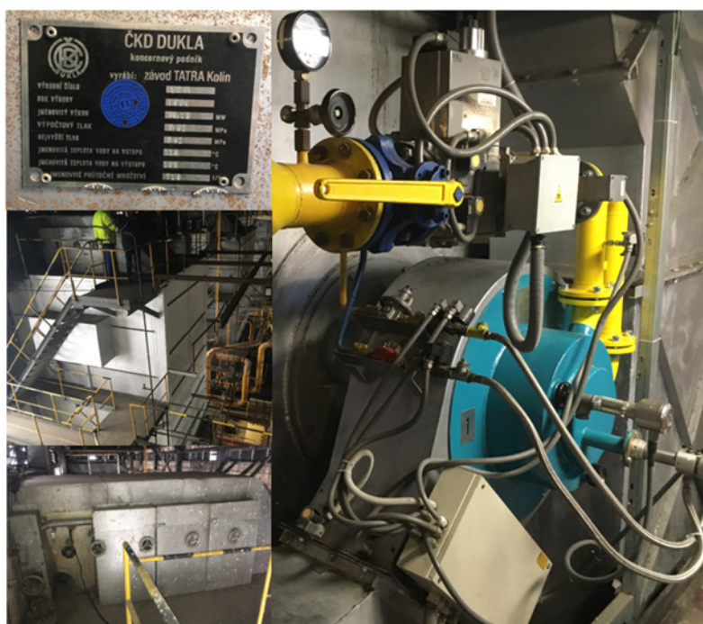
Figure 3. Boiler OK 60 ČKD Dukla. Clockwise: one of 4 gas burners; the top of the boiler duct; height view of the boiler; label with technical parameters of the boiler.
