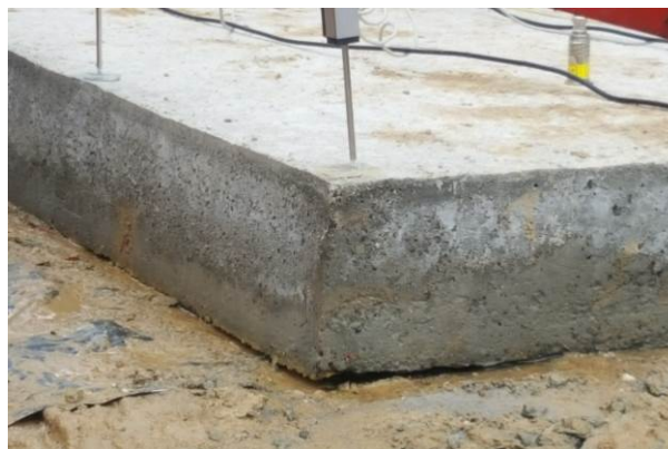
Fig. 25. Edge area of Concrete slab (after the test)
