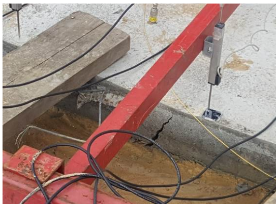
Fig. 24. Center area of the concrete slab – crack (after the test)
