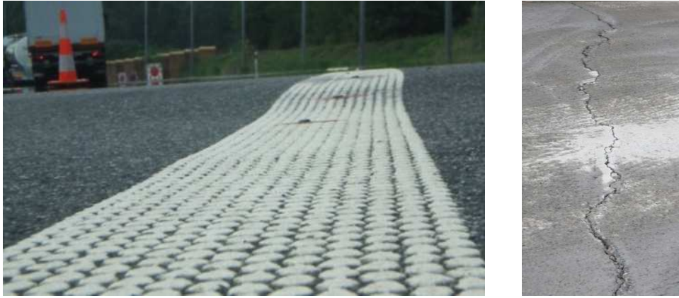
Fig. 3. Characteristic damage to road pavement in LDSA areas (Grygierek, 2017)
