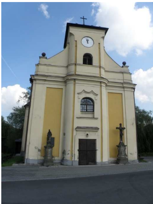
Fig.11 Church of St. Peter of Alcantara, the town of Karviná, Silesia, Czech Republic (sinking by 37 meters, leaning 6.8 degrees to the south); photo: Kaláb
