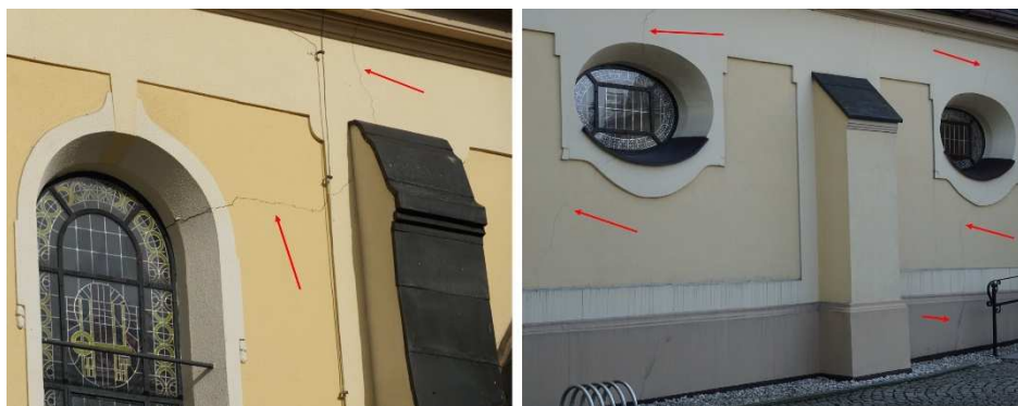
Fig.11 Fractures on the walls of the church; photo: Šcigala
