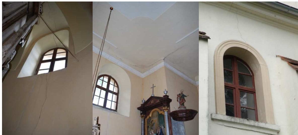
Fig. 2B Fractures of the walls and on the ceiling in the St. Andrew church; photo: Lednická
