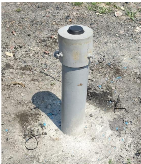
Figure 2 View of piezometer at point P-1, with wireless data recording
