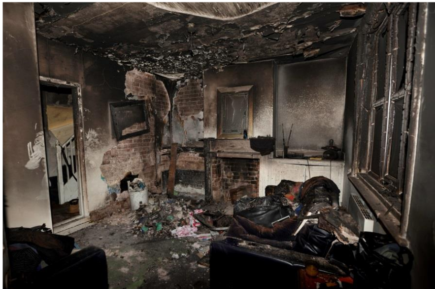
Fig. 8. The space after the fire (source: elaborated by authors)
