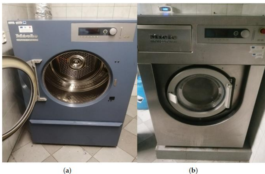
Fig. 10. (a) Dryer at the fire station; (b) Washing machine at the fire station (source: elaborated by authors)
