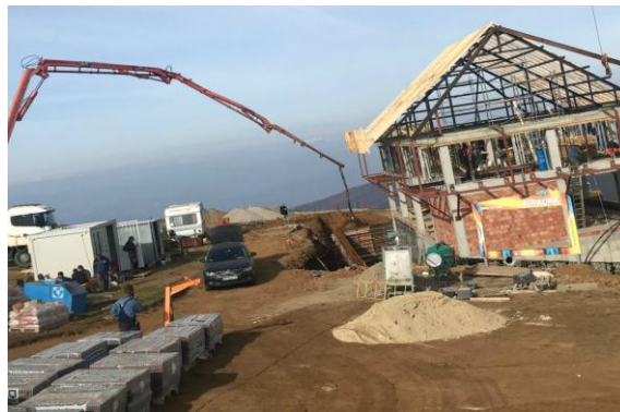
Fig. 2. Illegal construction activities on Kopaonik
